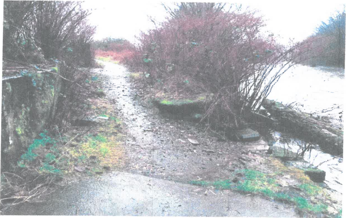
Figure 1: Flooding of entire path where it passes under railway bridge.
